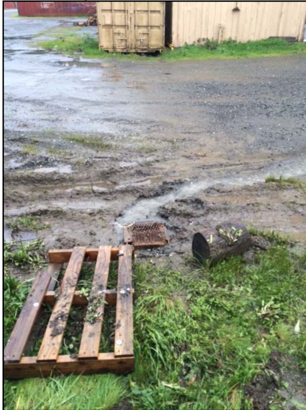
Figure 4.2A Drainage Inlet on the Elevated Portion of the Site
