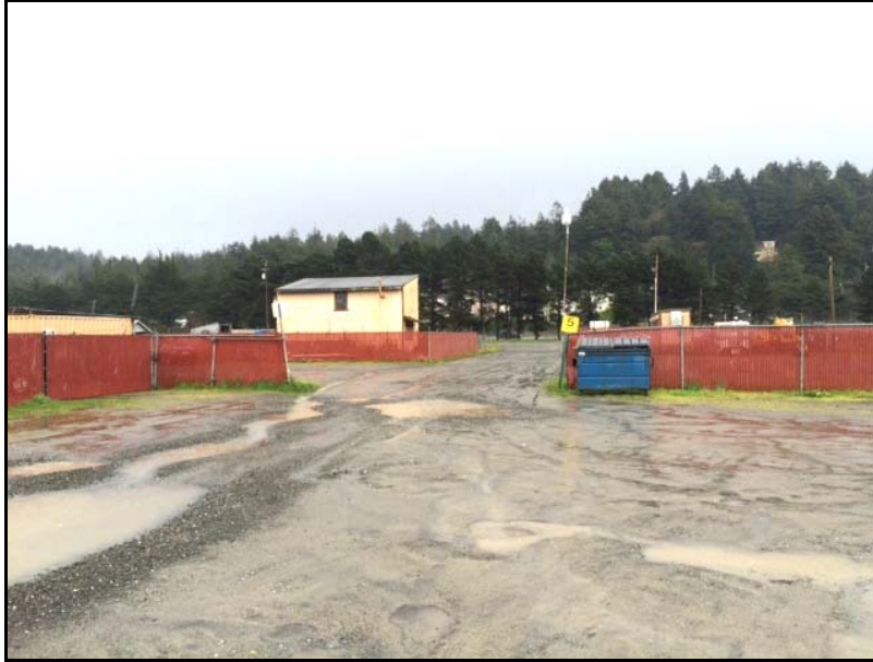
Figure 4.2C Ponding of Water on the Elevated Portion of the Site
