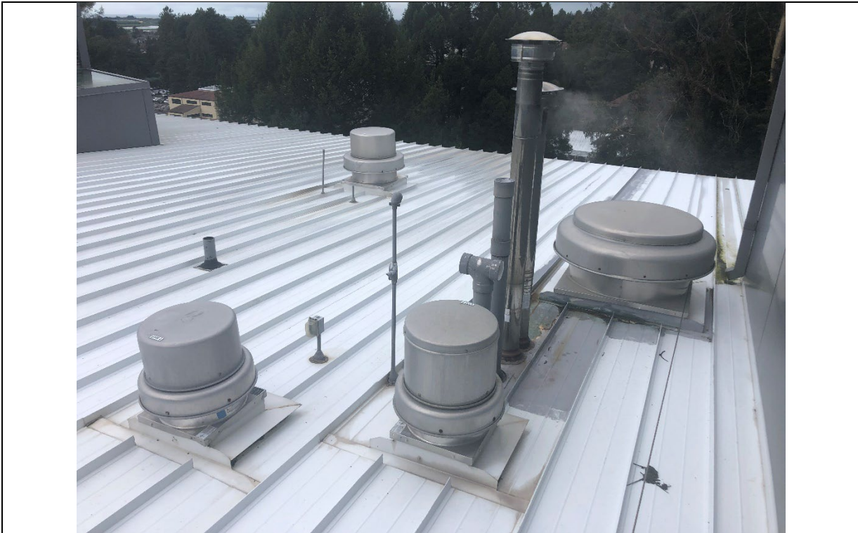
Photograph 5 – BSS Building – Roof Exhaust
