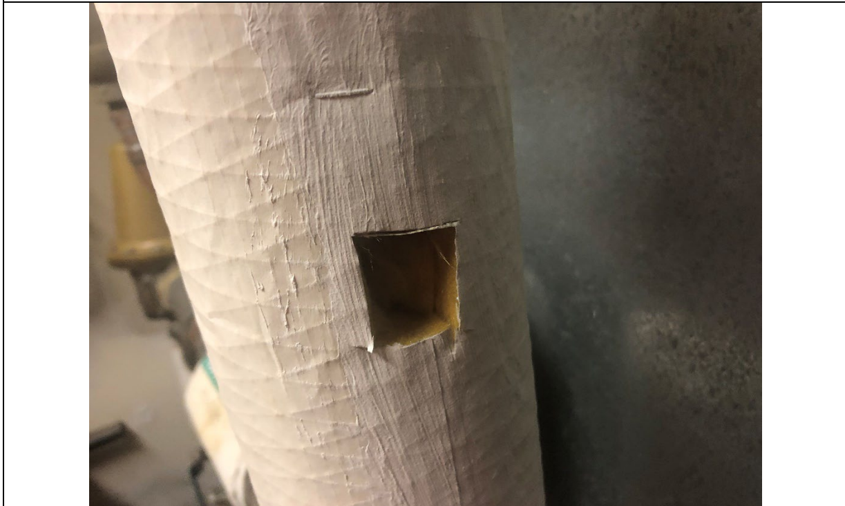
Photograph 4 – BSS Building – Room M-0B – Fiberglass TSI Run (Typical)
