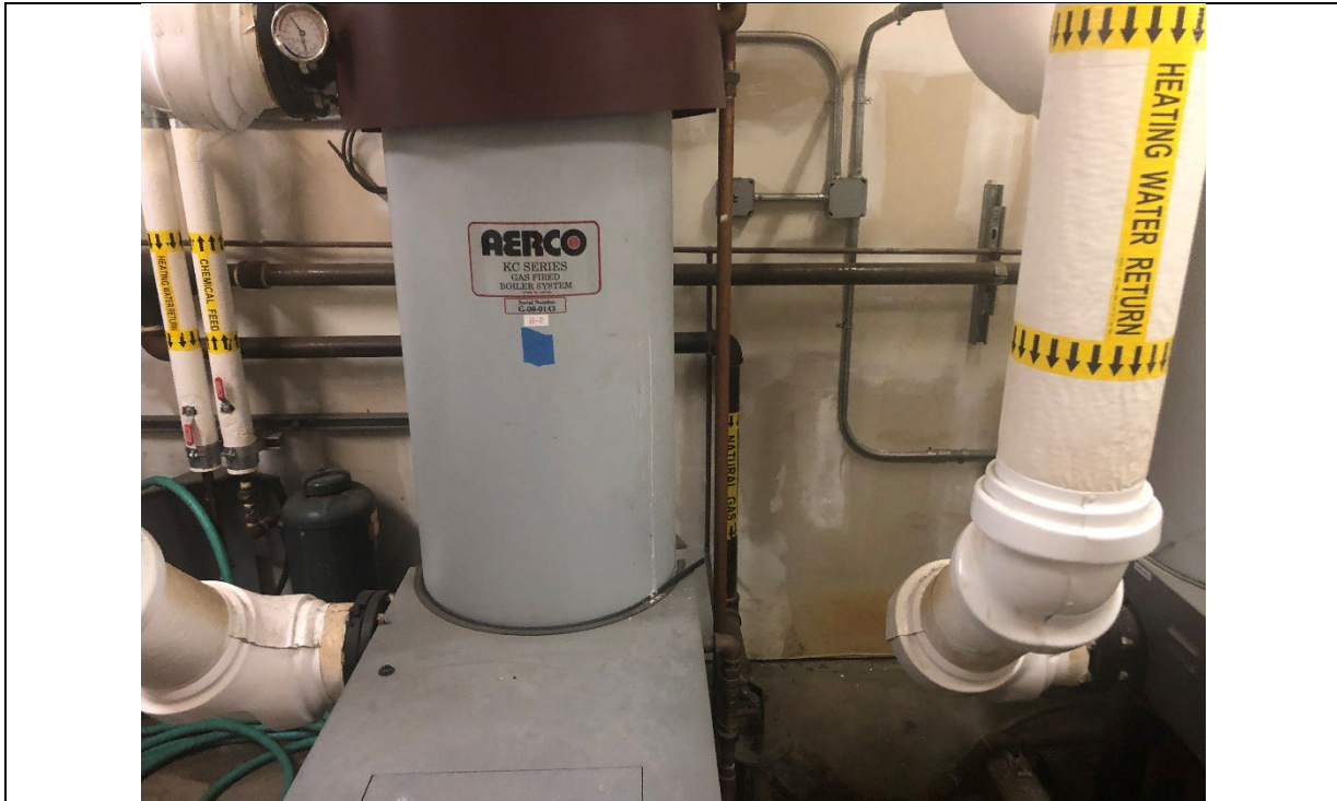
Photograph 3 – BSS Building – Room M-0B Vertical TSI and 45° Fitting (Typical)
