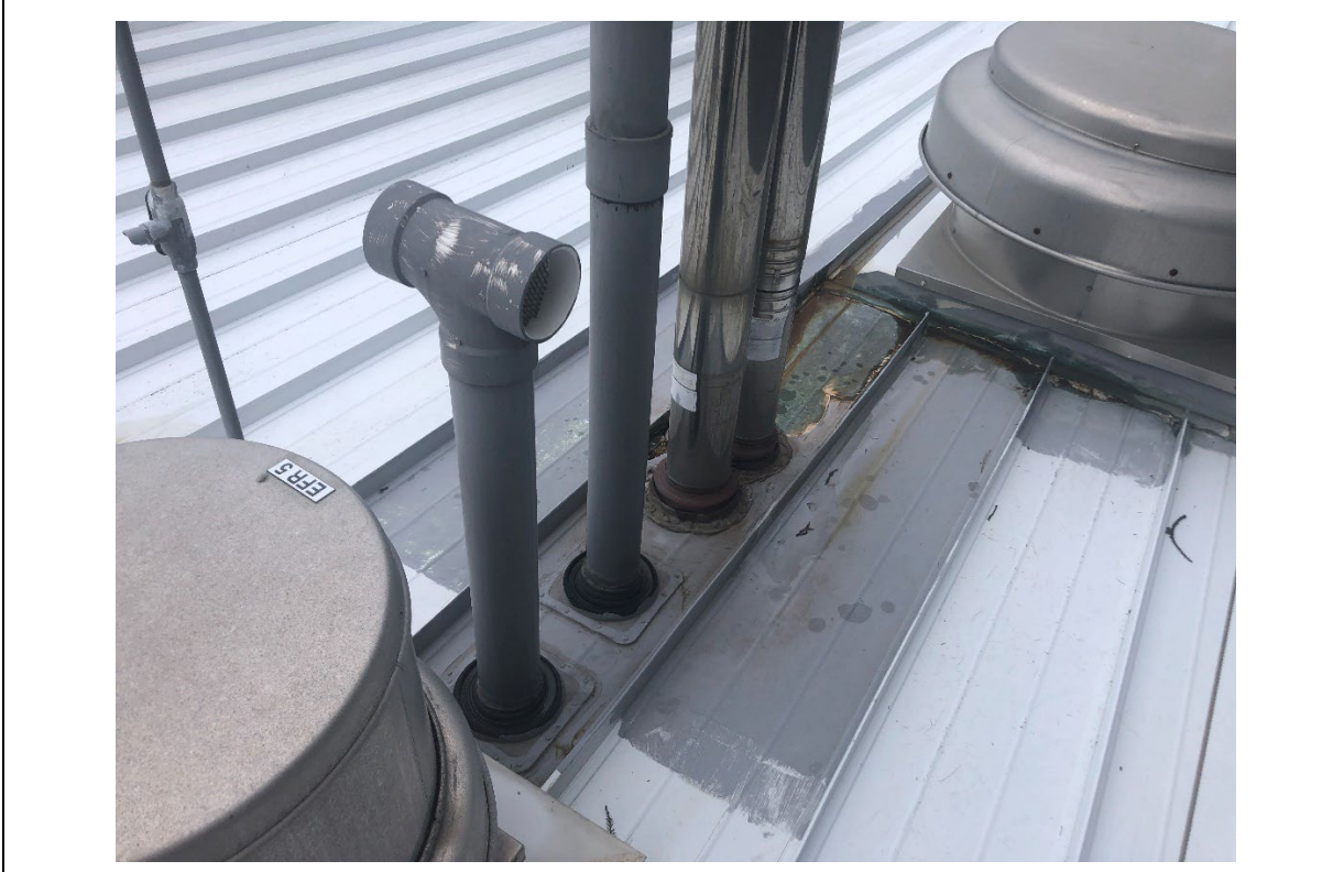
Photograph 6 – BSS Building – Roof Exhaust Detail
