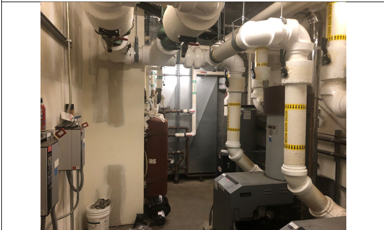
Photograph 2 – BSS Building – Room M-0B Horizontal and Vertical TSI Typical
