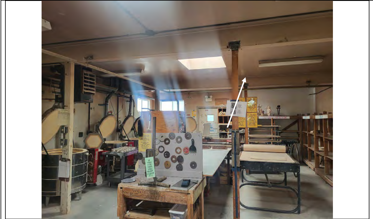
Photograph 9 – CERAM Interior – Drywall and joint compound walls and ceiling (typical) reported to contain asbestos
