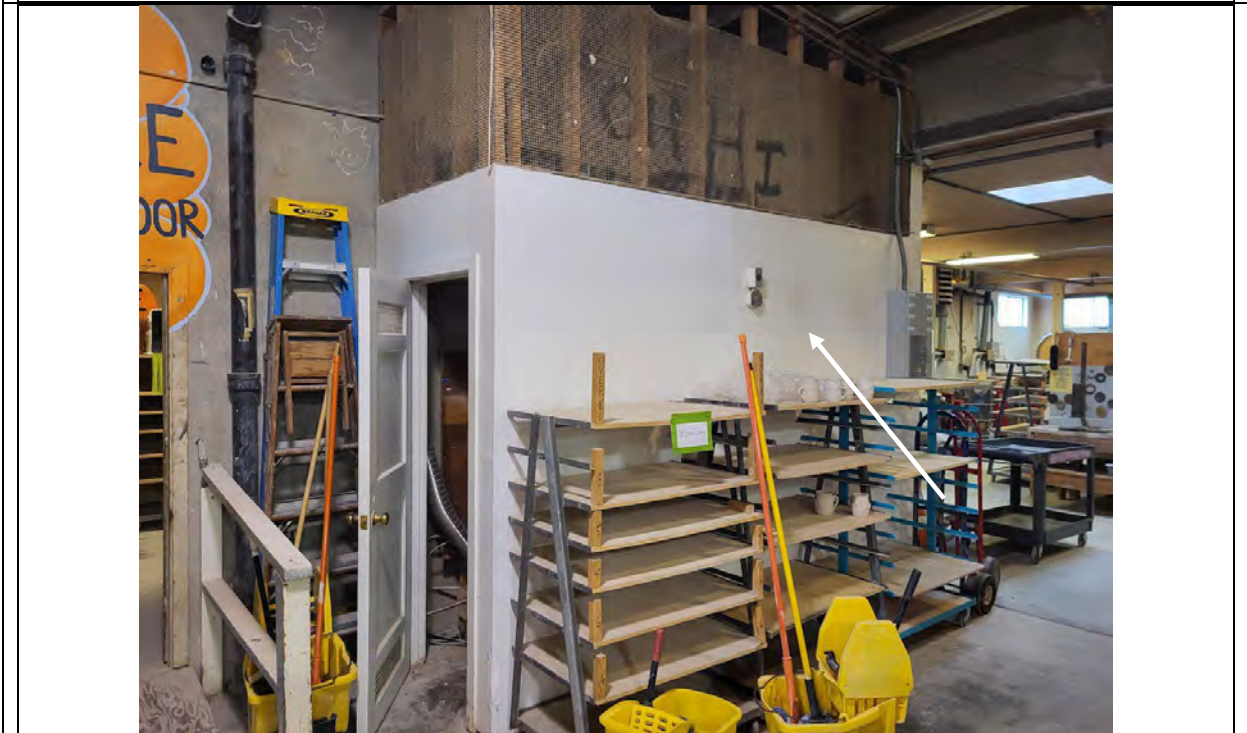
Photograph 10 – CERAM Interior – Drywall and joint compound wall (typical) reported to contain asbestos
