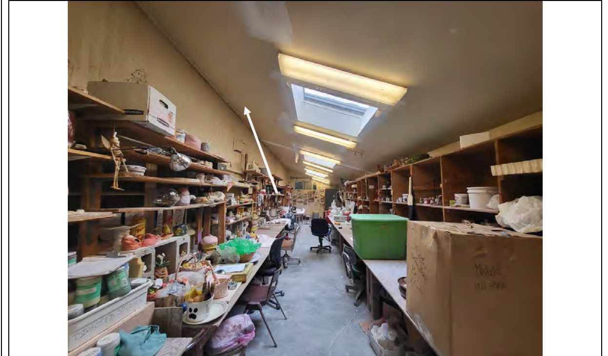
Photograph 8 – CERAM Interior – Drywall and joint compound walls and ceiling (typical) reported to contain asbestos
