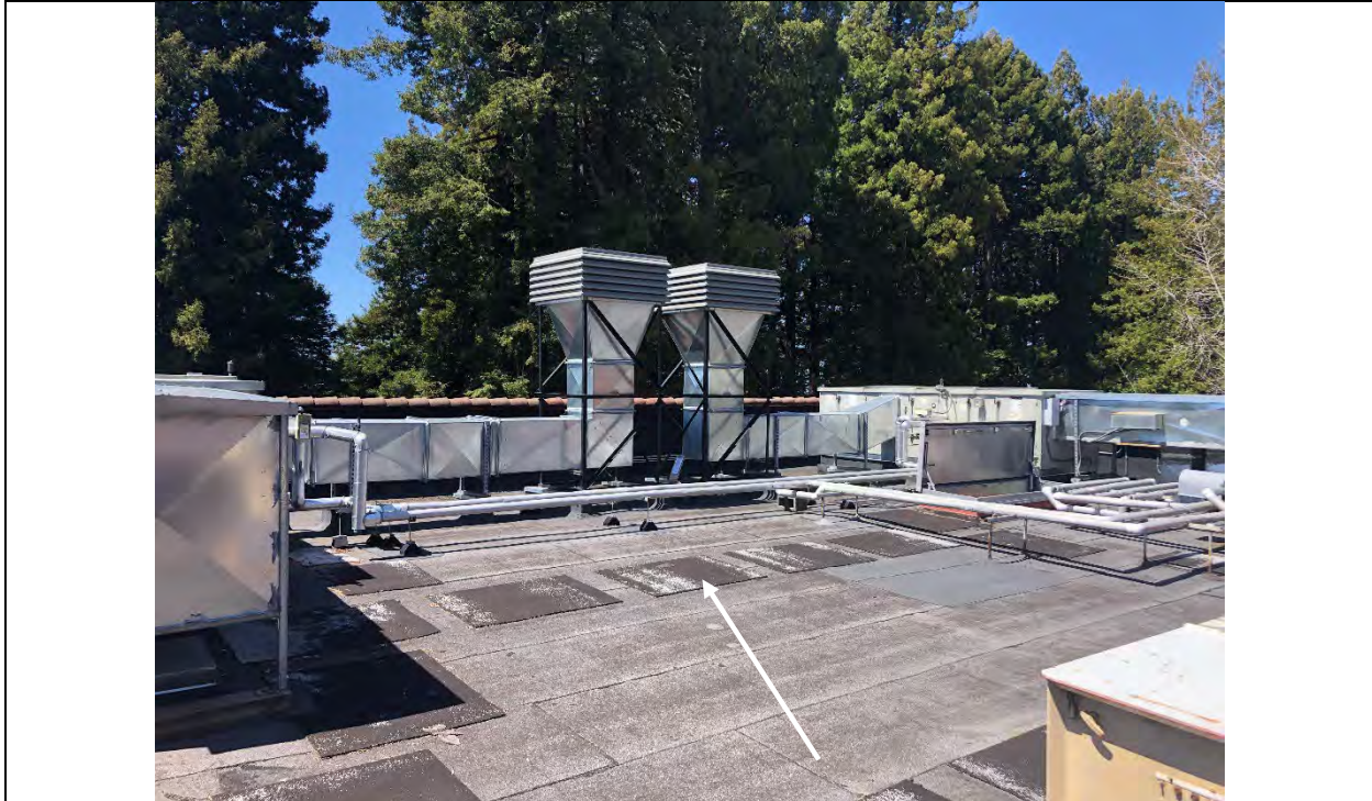
Photograph 1 – SHC Roof – Mastic associated with underside of walking pads reported to be ACM (note: walk pad is nondetect)
