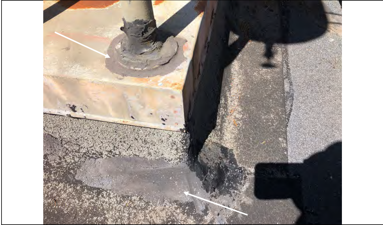
Photograph 3 – SHC Roof – Roof mastic (typical) homogeneous with material reported to be ACM
