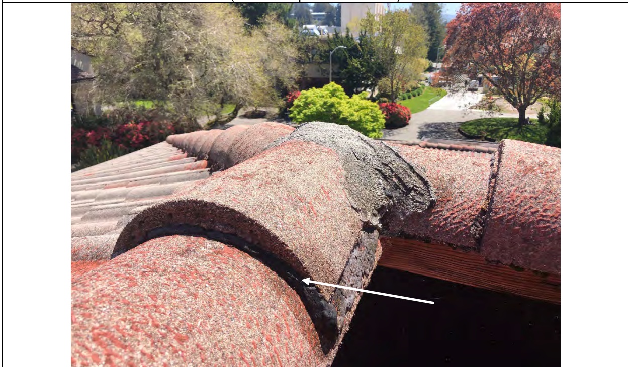
Photograph 2 – SHC Roof – Roof mastic (typical) at parapet tile reported to be ACM (note: cement patch material is nondetect)
