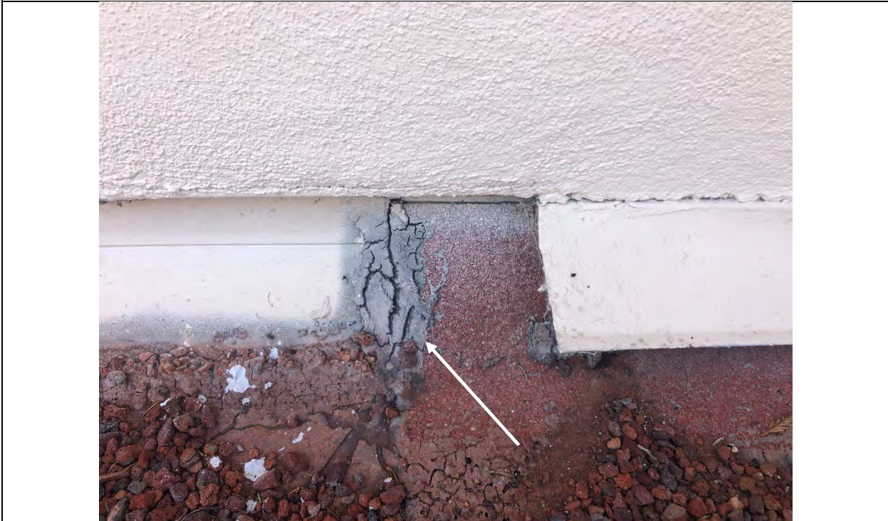
Photograph 4 – GSAC Roof – Roof mastic (typical) at seams and penetrations reported to be ACM
