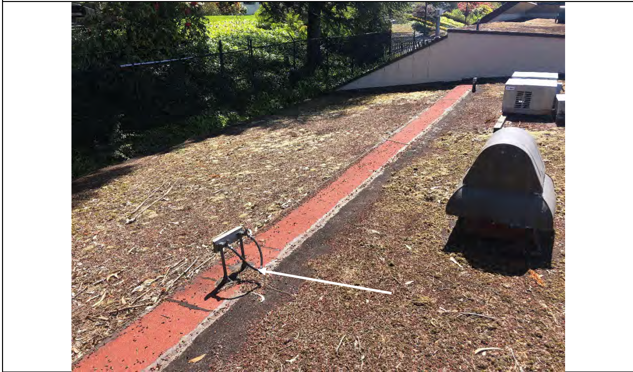
Photograph 2 – GSAC Roof – Roof mastic (typical) at seams and penetrations reported to be ACM
