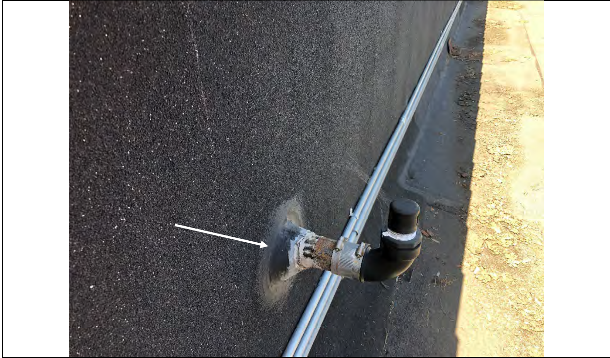
Photograph 5 – SHC Roof – Roof mastic (typical) homogeneous with material reported to be ACM
