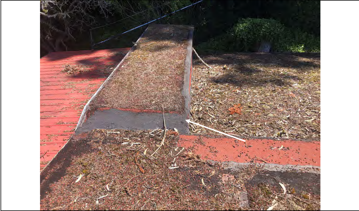
Photograph 3 – GSAC Roof – Roof mastic (typical) at seams and penetrations reported to be ACM
