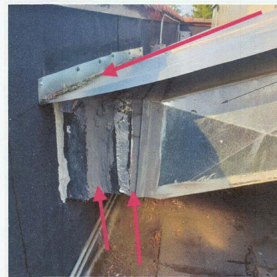
TYPICAL DUCTWORK CONDITION
