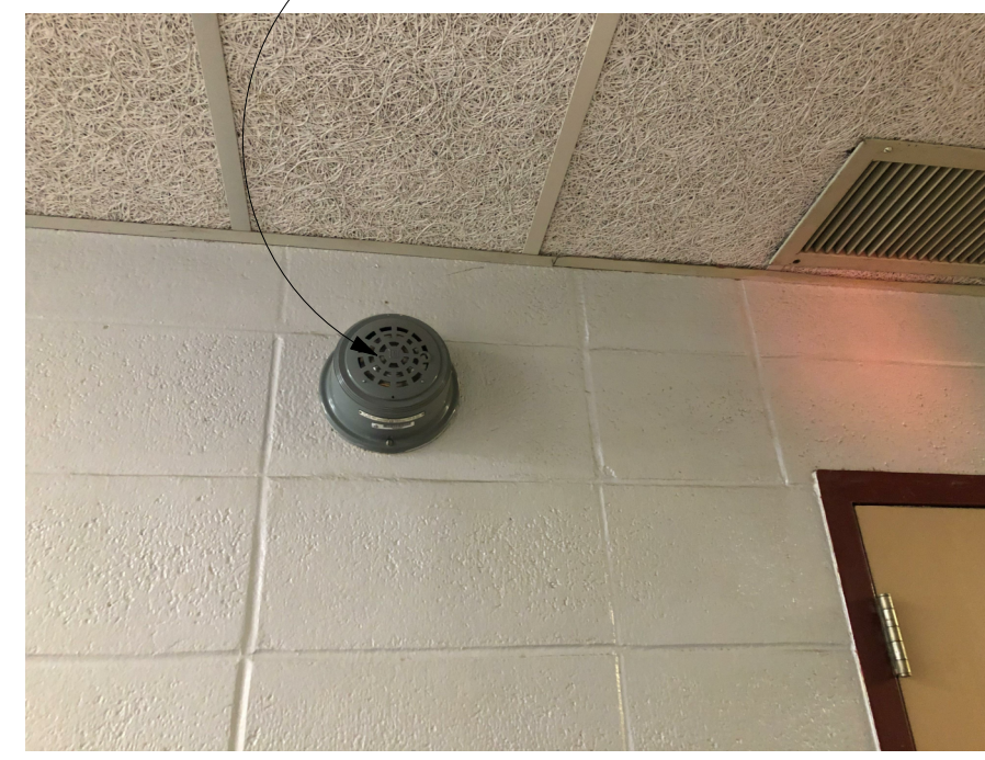
3 S - PHOTO @ (E) FIRE ALARM HORN 1/8" = 1'-0"
