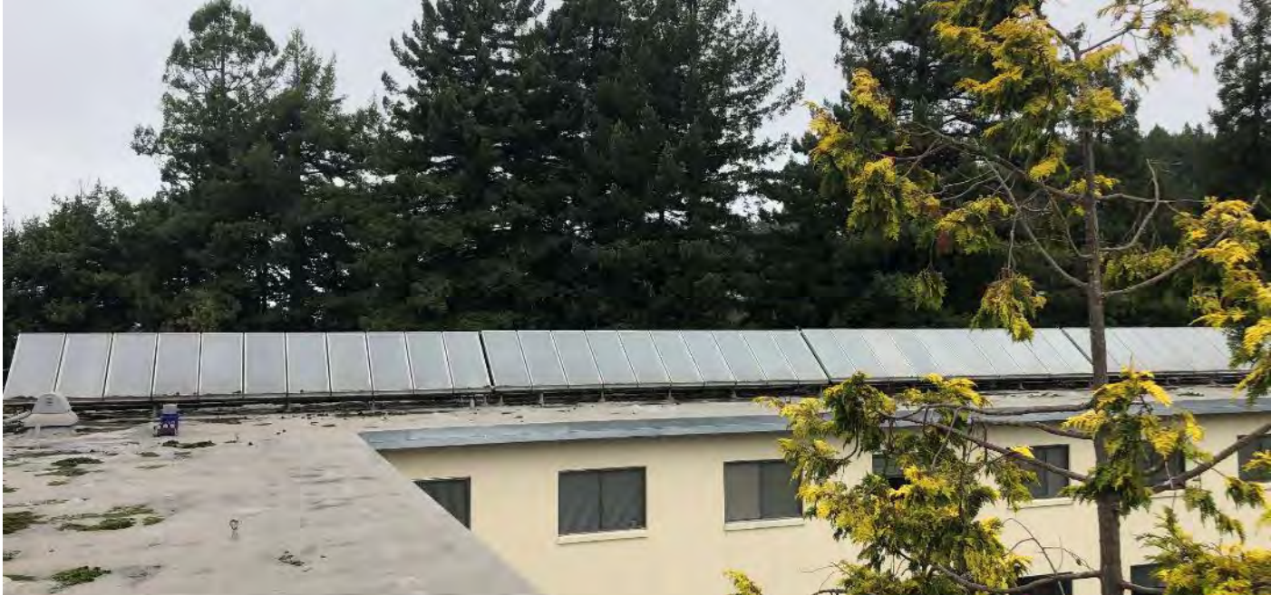
Photo 1 Main Roof – North and East wing roofs with solar hot water panels
