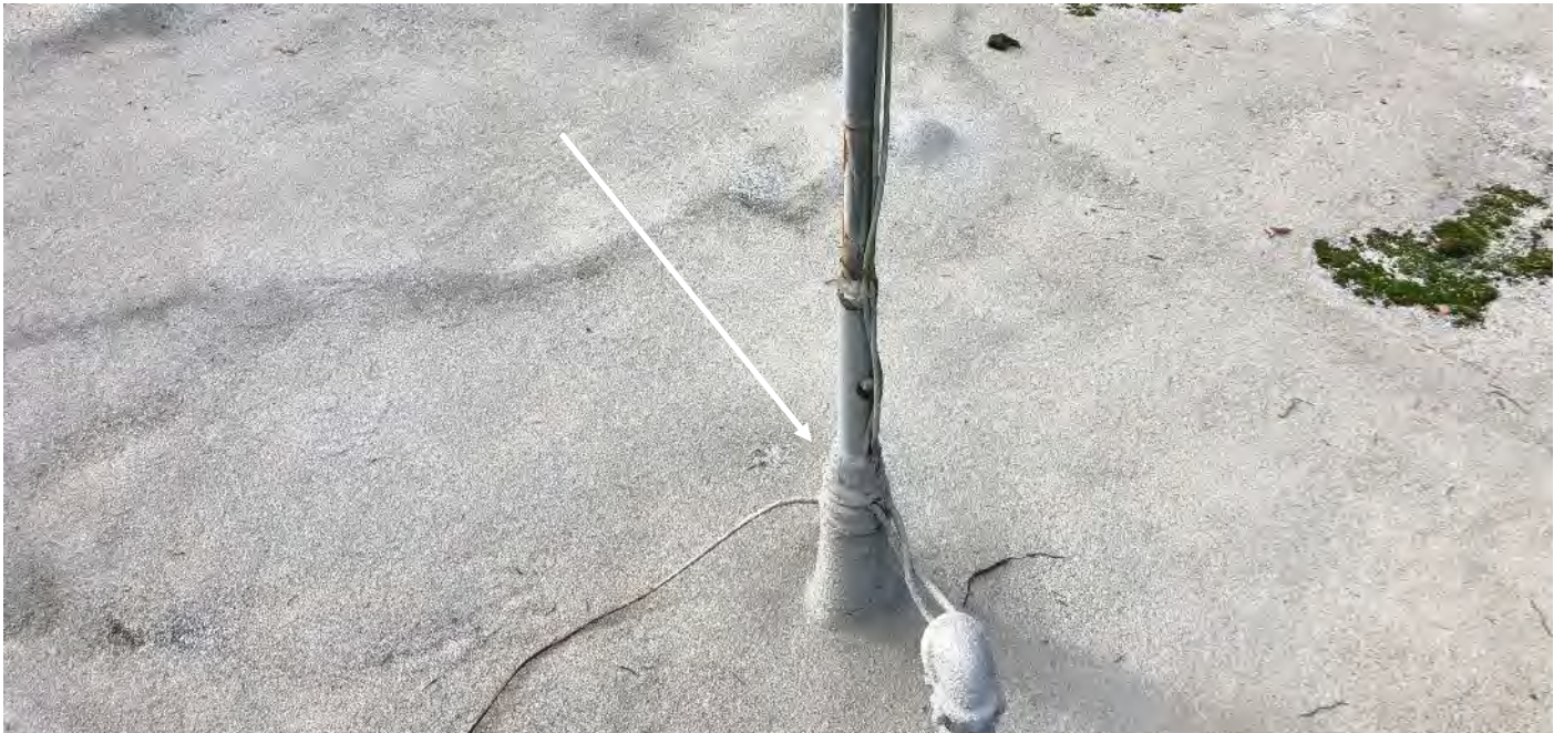
Photo 3 Main roof – Penetration caulk (white/grey) at penetrations (typical indicated by arrow) reported to contain asbestos
