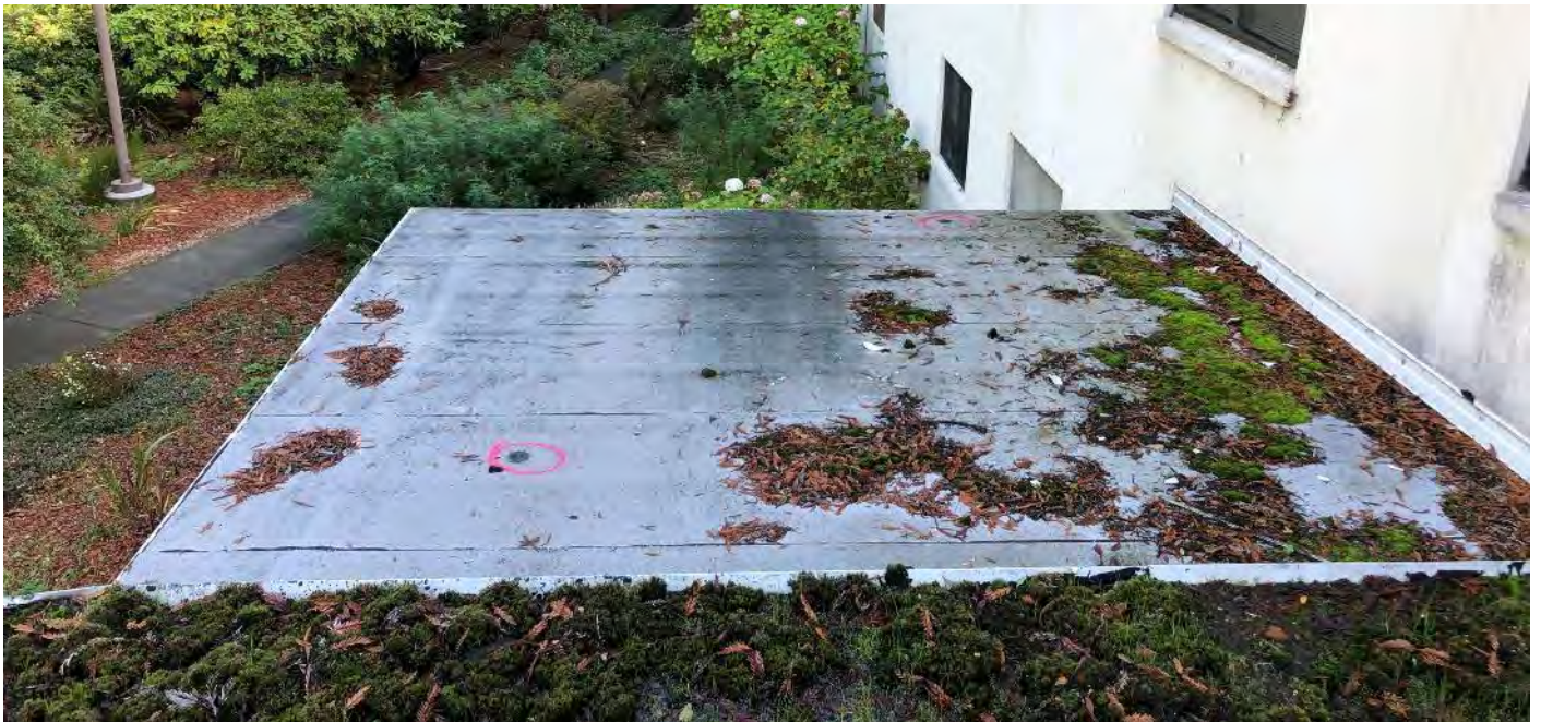
Photo 8 Northeast Addition Roof (NE Roof) – Rolled roofing system reported to be nondetect for asbestos
