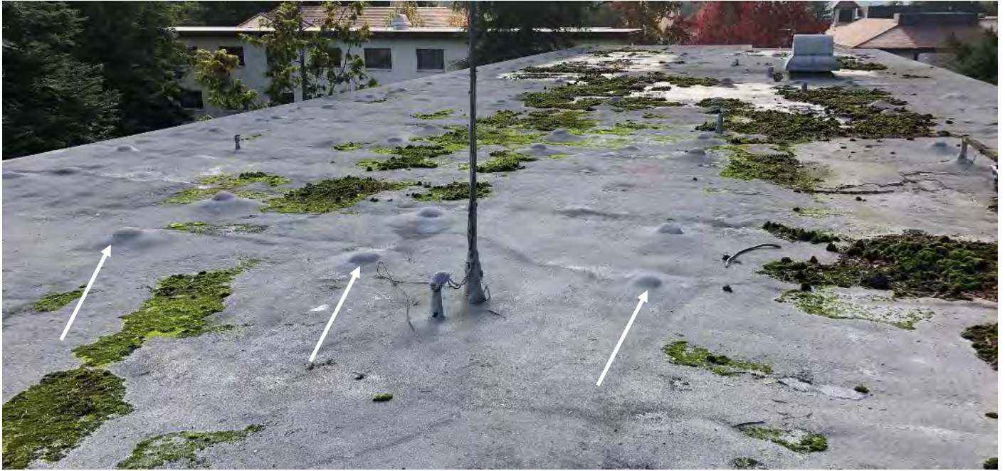
Photo 5 Main roof – Roofing mastic (not shown, location typical) at remanent footers reported to contain asbestos
