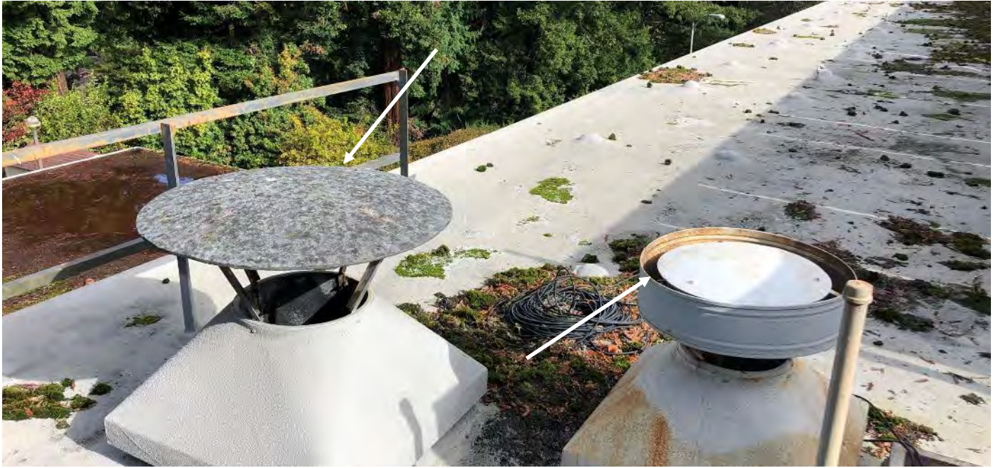
Photo 7 Main roof – HVAC vents at NE corner – Vent caps (indicated by arrows) reported to contain asbestos
