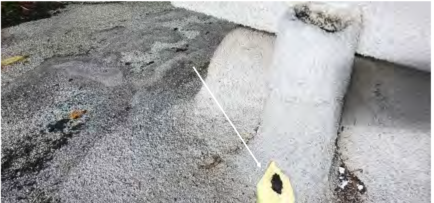
Photo 4 Main Roof – Roof mastic (black), indicated by arrow, reported to contain asbestos (foam coating [grey/cream] is nondetect for asbestos)
