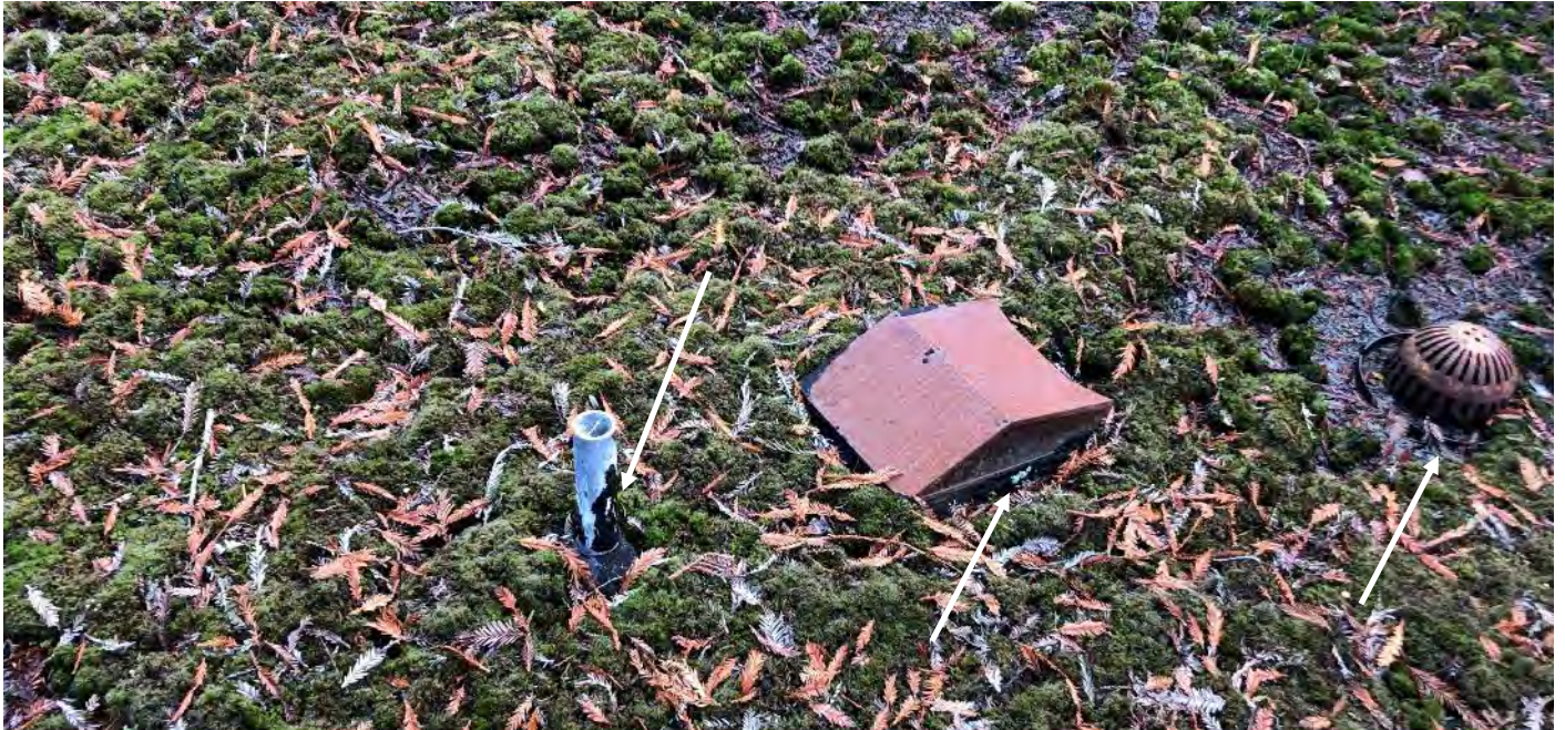
Photo 10 Lower Roof (L1) – Roof mastic (black) (typical) associated with building exterior walls reported to contain asbestos
