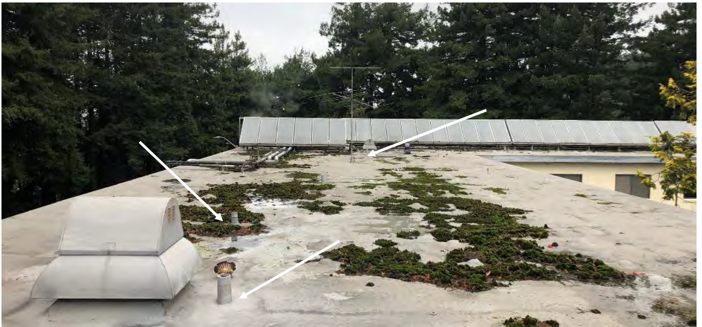
Photo 2 Main roof – Roofing mastic at penetrations (typical indicated by arrow), vents, and equipment footers reported to contain asbestos
