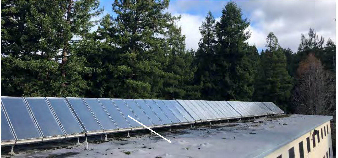
Photo 6 Main roof – Roofing mastic at former footers (typical indicated by arrow) reported to contain asbestos
