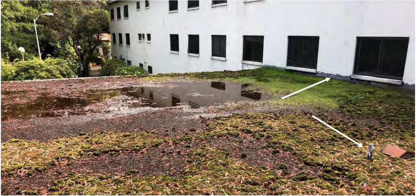
Photo 9 Lower Roof (L1) – Roof mastic (black) associated building exterior wall and roof penetrations (typical location indicated by arrows) reported to contain asbestos
