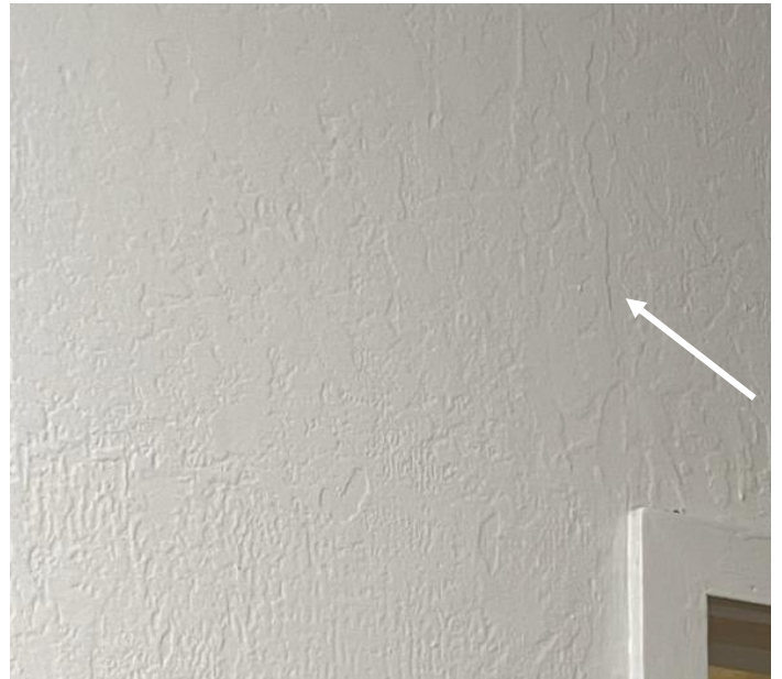
Photo 4 Maple – Third Level Corridor – Knock down surface texture (indicated by arrow, typical) associated with drywall wall and ceiling systems reported to contain asbestos.
