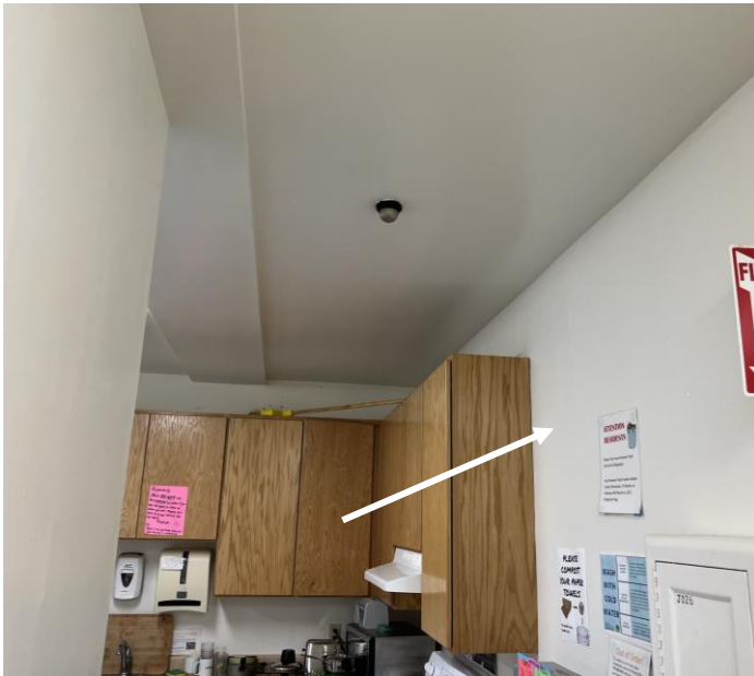
Photo 7 Maple – Basement Kitchen Area – Drywall/joint compound wall and ceiling systems (indicated by arrow) associated with smooth surface coating reported to be nondetect for asbestos.
