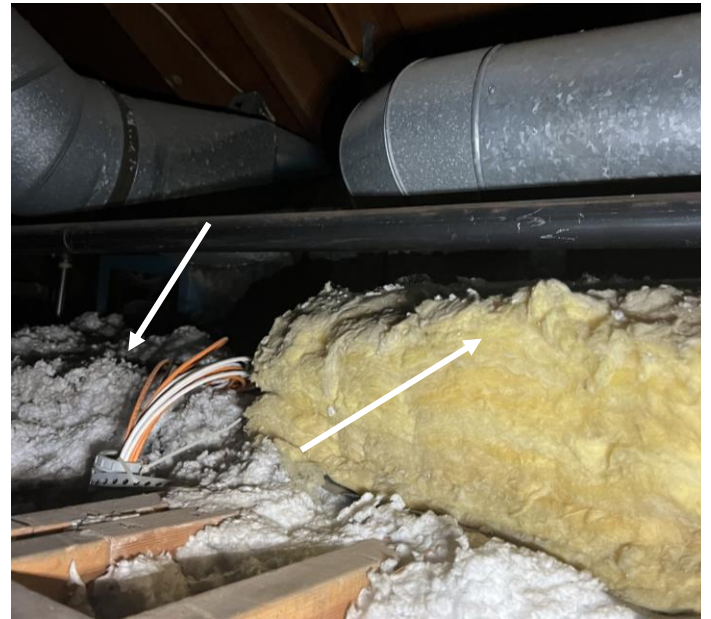
Photo 8 Maple – Third Level Attic/Crawlspace – Blown-in insulation (white) and batt insulation (yellow) were both reported as nondetect for asbestos.
