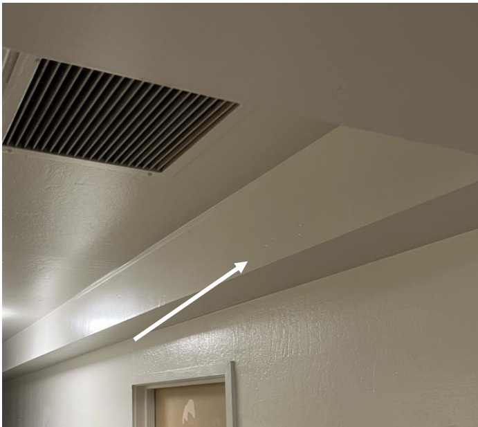
Photo 3 Hemlock – First Level Corridor – Drywall/joint compound wall and ceiling systems, including at soffit (indicated by arrow) reported to contain asbestos.
