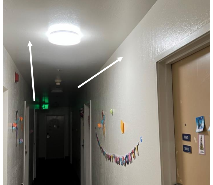
Photo 2 Hemlock – Third Level Corridor – Drywall/joint compound wall and ceiling systems (indicated by arrow, typical for project site) reported to contain asbestos.
