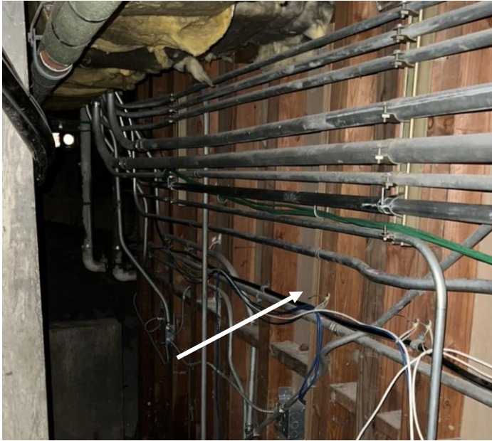
Photo 5 Hemlock – Basement Crawlspace – Drywall/joint compound wall and ceiling systems (indicated by arrow) reported to contain asbestos.
